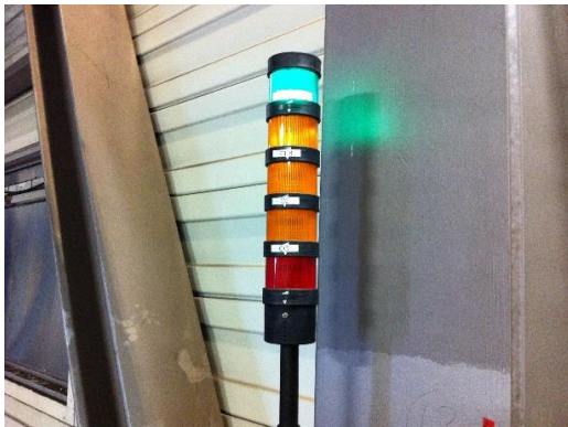
Figure 6 Warning Signs at the entrance of the silo
