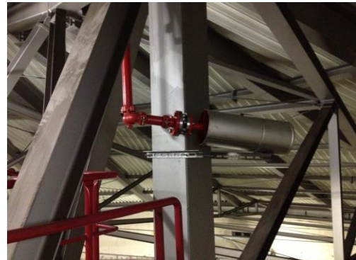
Figure 7 Foam Thrower in top of silo
