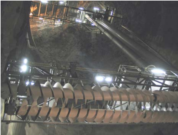
Fig. 7. View of the underground Eurosilo®
